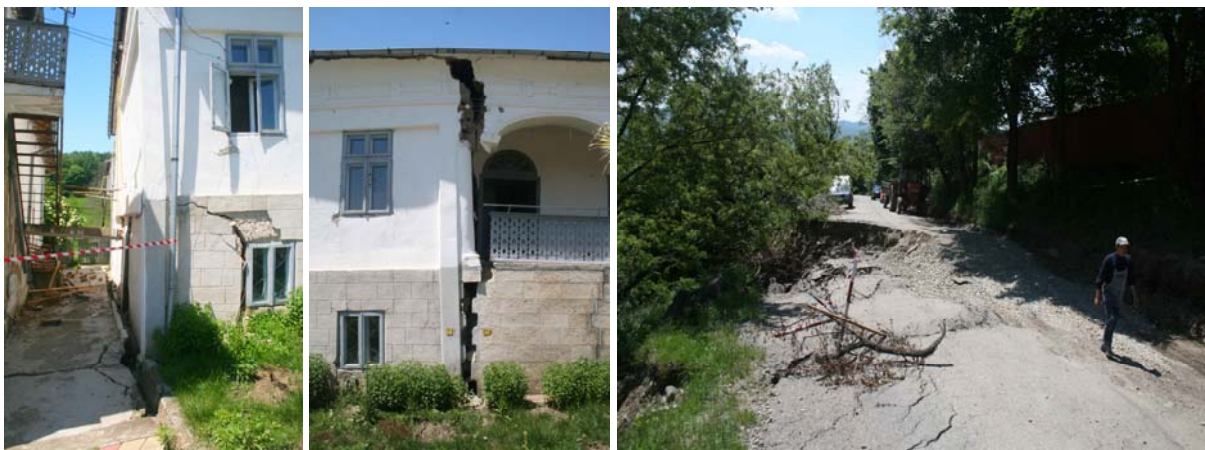
Fig. 4. Rătești monastery, affected by a landslide in June 2014
